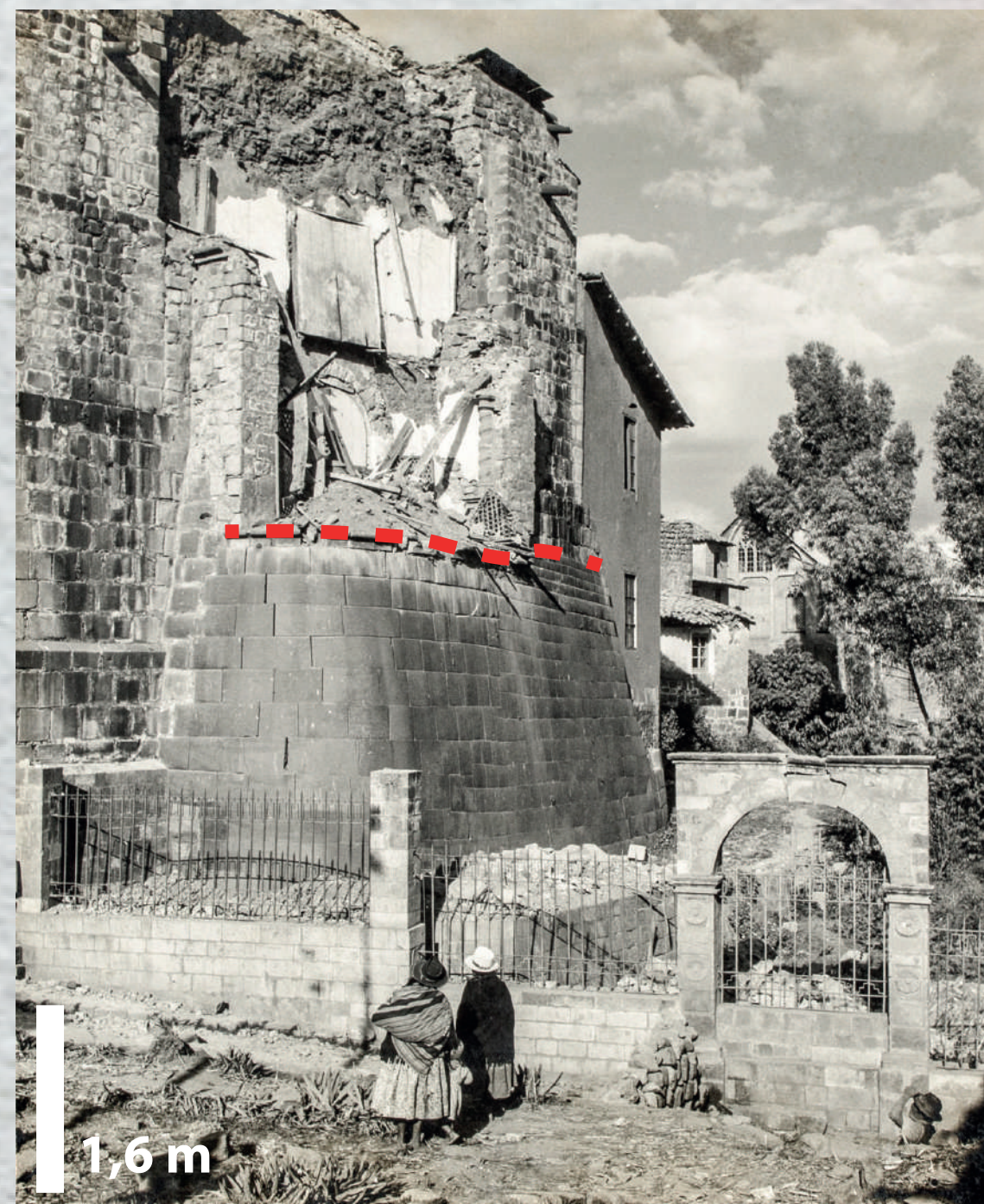
Fig.I Picture of the Santo Domingo convent (Qorikancha) in Cuzco after the 1950 earthquake. Credits: LIFE
