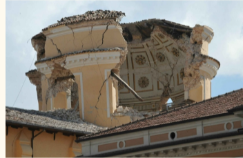
Church, L'Aquila earthquake, 2009, Italy [Limoge, 2016]
